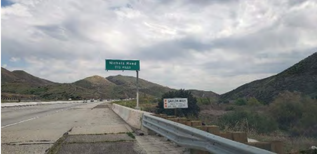
Site 34 – Bridge Maintenance on I-15 PM 25.55 Over Gavillan Wash Project (now Gavillon Wash Bridge) ( I-15 PM 25.55, Lake Elsinore, California). Photo facing south east.
