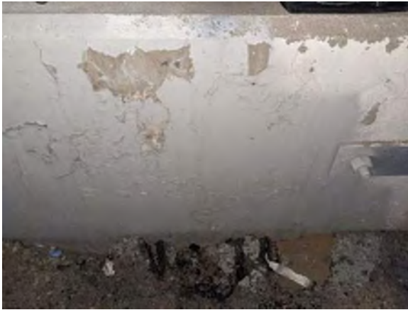
View of Light Gray Paint on 56-0680R – Northbound Temescal Wash, Inside Rail
