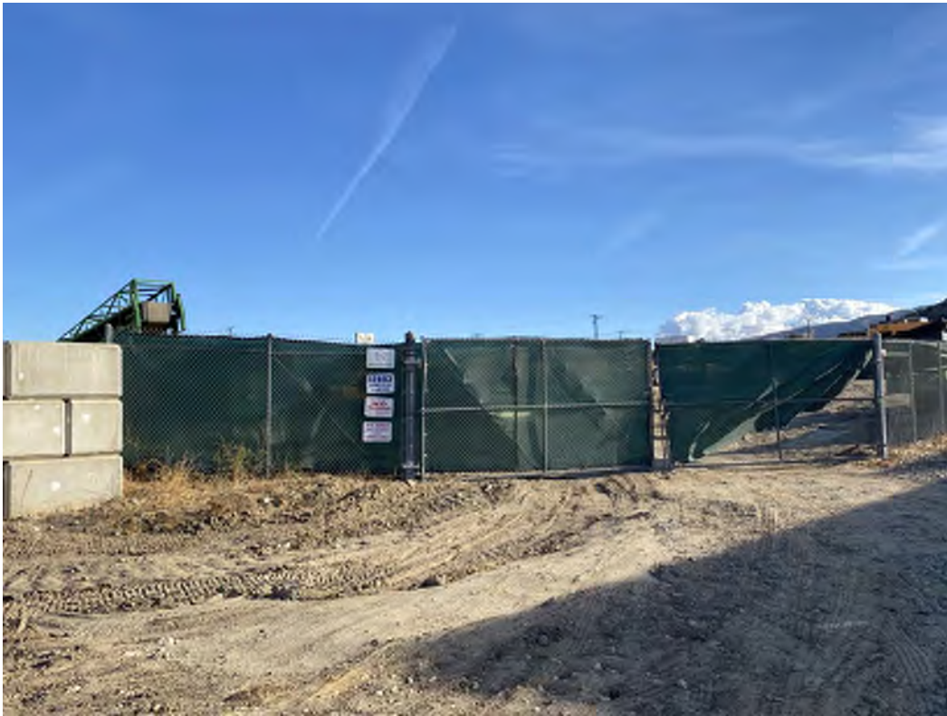
Site 44 – Temescal Canyon Compost Facility (12893 Temescal Canyon Road, Corona, California). Photo facing southeast.
