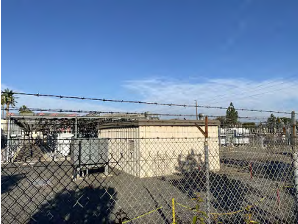
Site 95 – SCE Chase Substation (1390 E. Ontario Avenue, Corona, California). Photo facing northwest.
